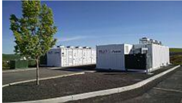
1 MW 4 MWh containerized vanadium flow battery owned by Avista Utilities and manufactured by UniEnergy Technologies
