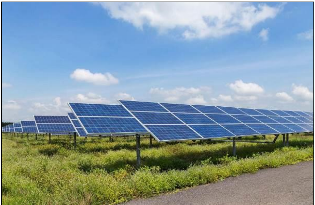
Photograph 1.1: Typical PV SEF facility
