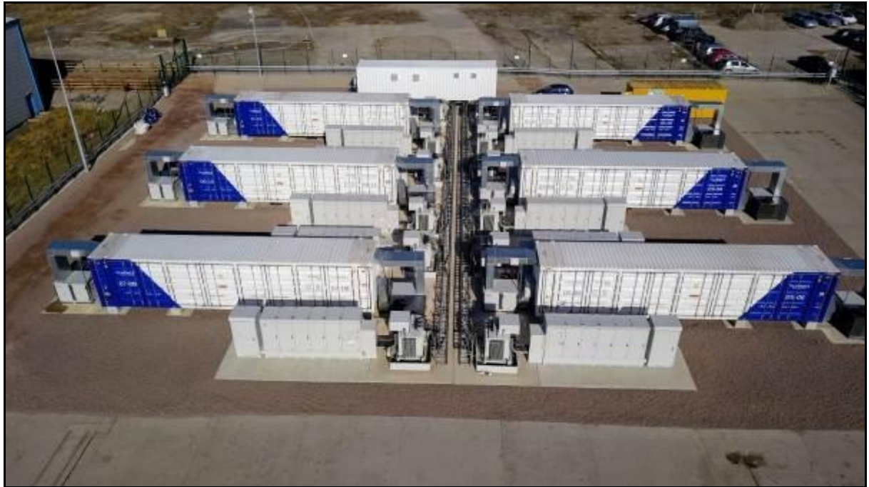
Photograph 1.2: Example of BESS located in storage containers
