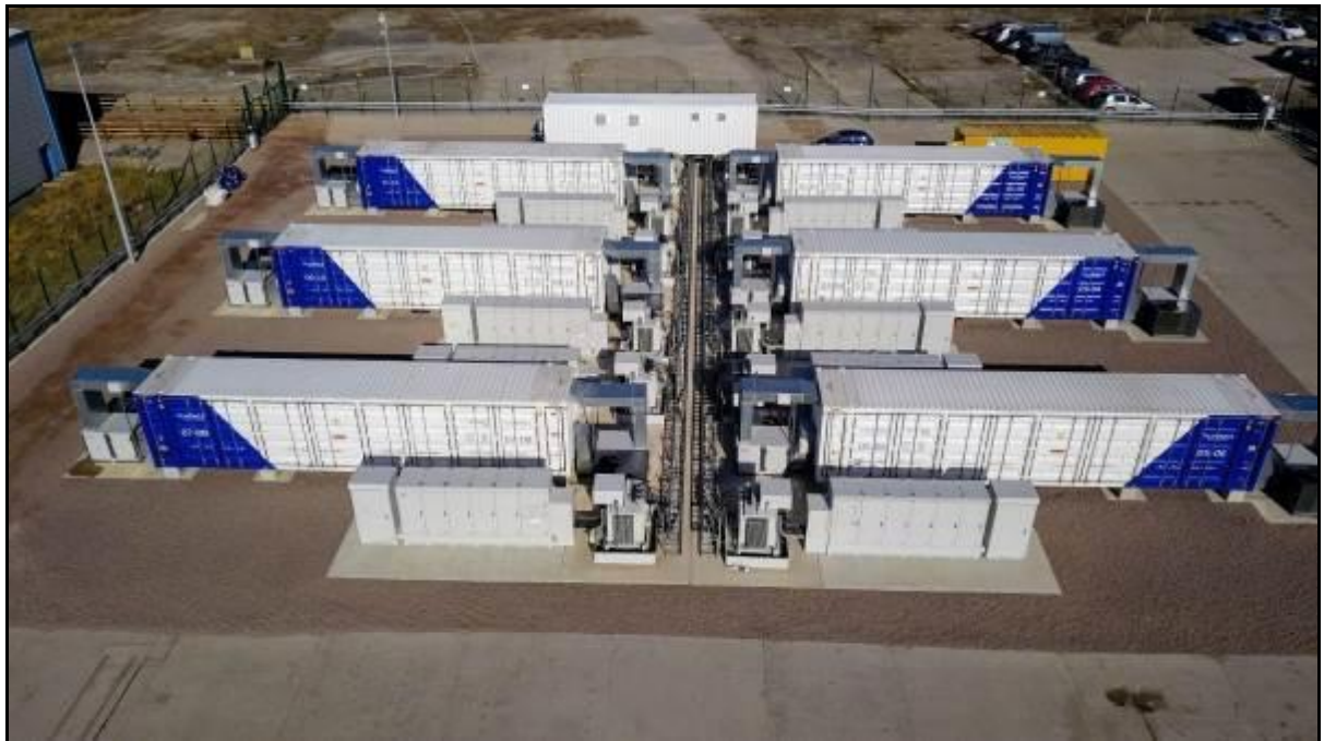
Photograph 1.2: Example of BESS located in storage containers
