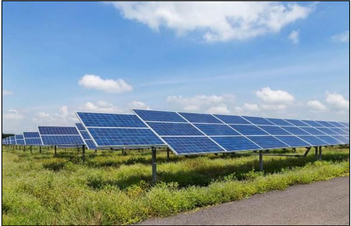
Photograph 1.1: Typical PV SEF facility
