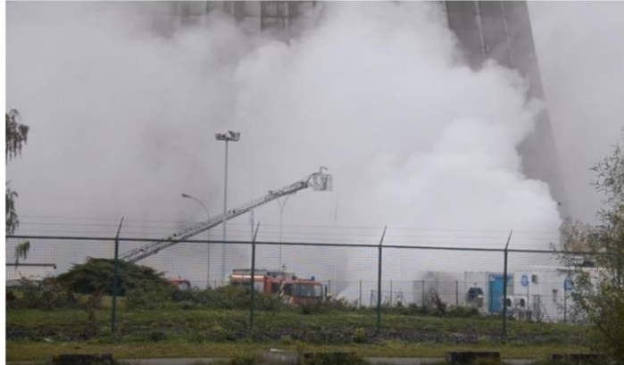
A fire engulfs a lithium-ion battery system at an Engie test site in Belgium, Nov. 11.
