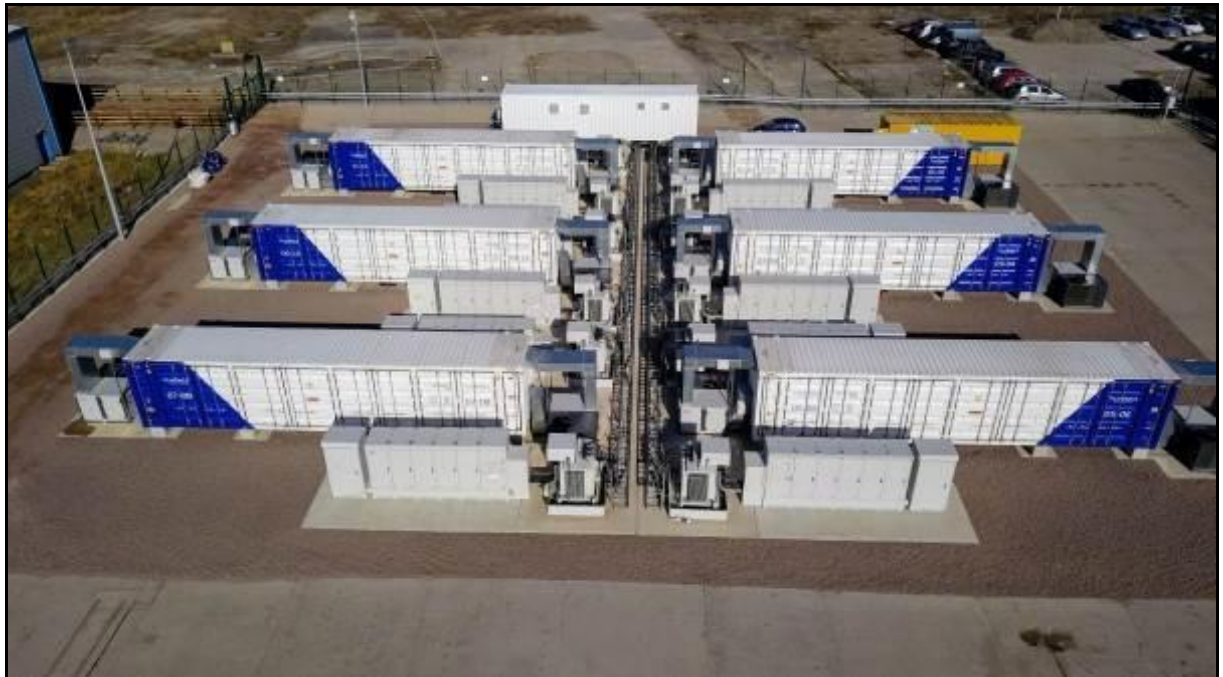
Photograph 1.2: Example of BESS located in storage containers
