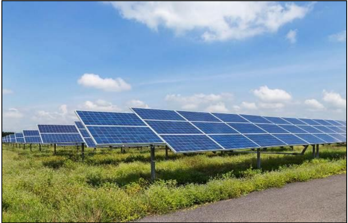
Photograph 1.1: Typical PV SEF facility
