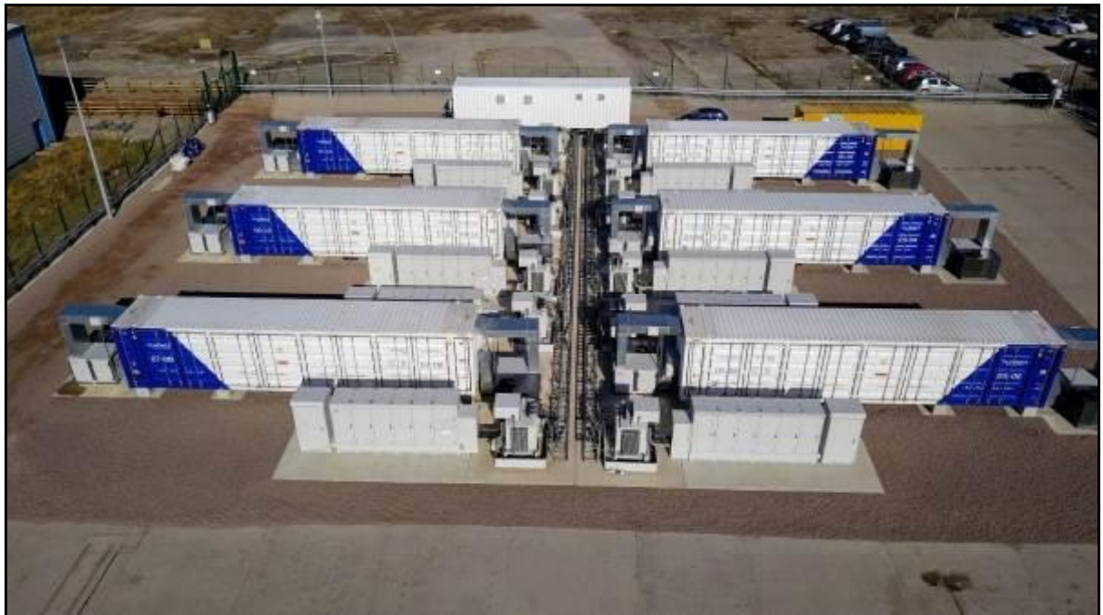
Photograph 1.2: Example of BESS located in storage containers
