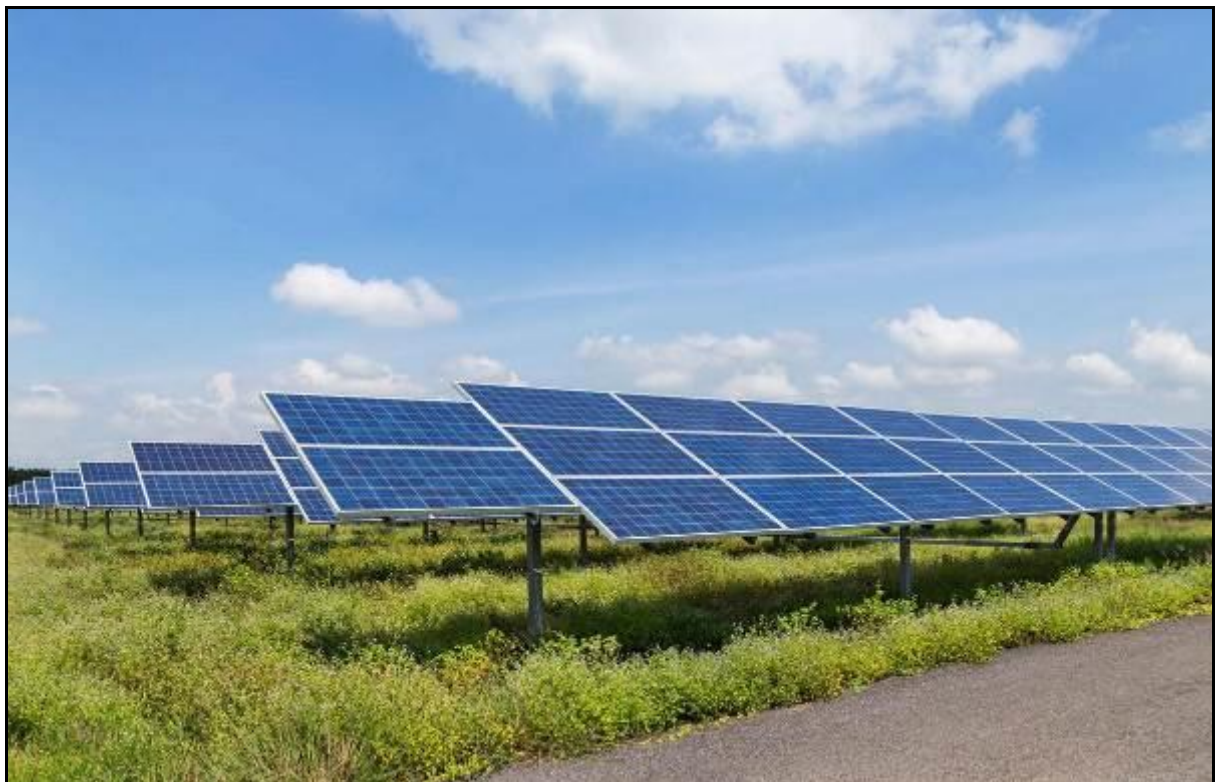
Photograph 1.1: Typical PV SEF facility
