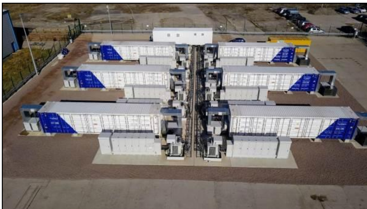
Photograph 1.2: Example of BESS located in storage containers
