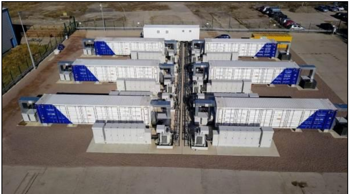
Photograph 1.2: Example of BESS located in storage containers
