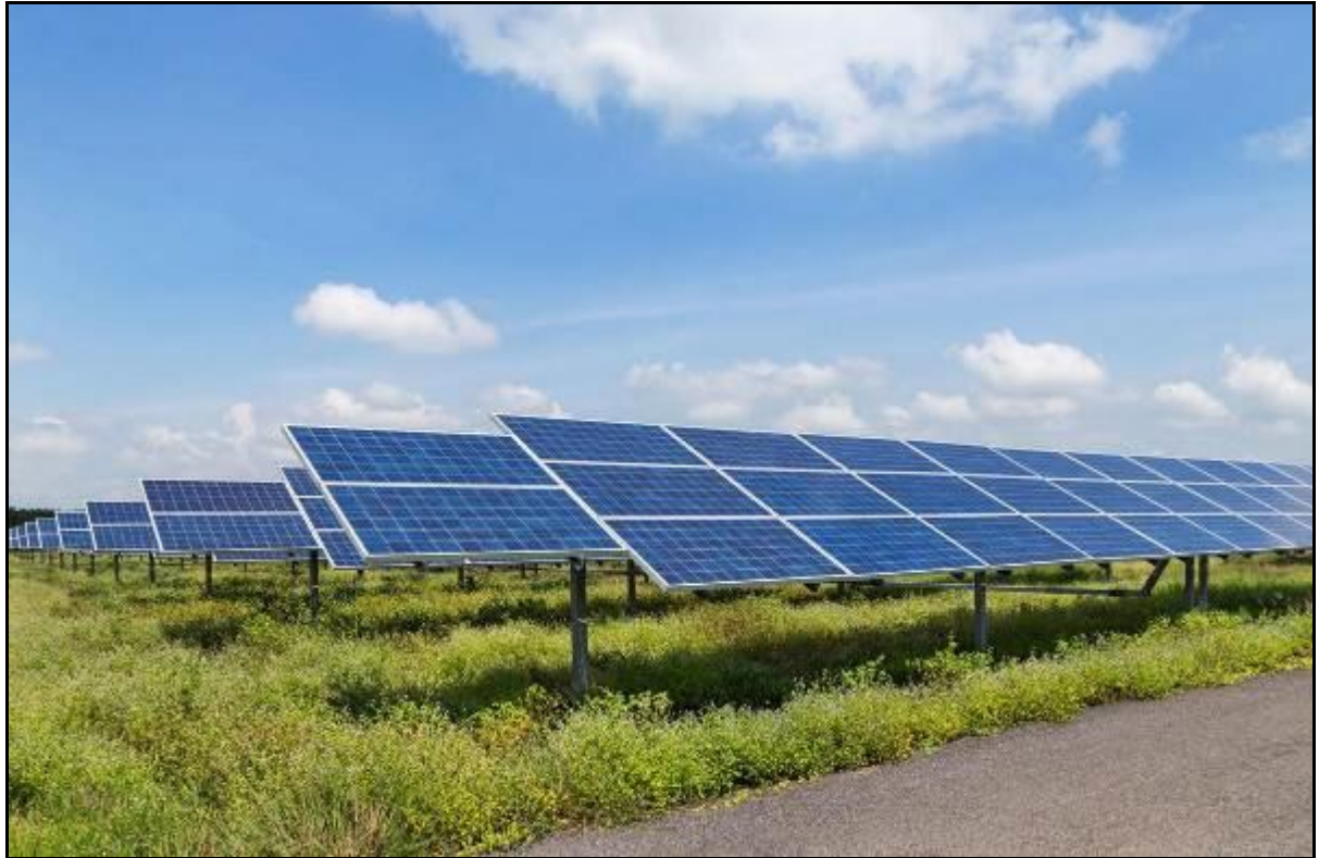
Photograph 1.1: Typical PV SEF facility
