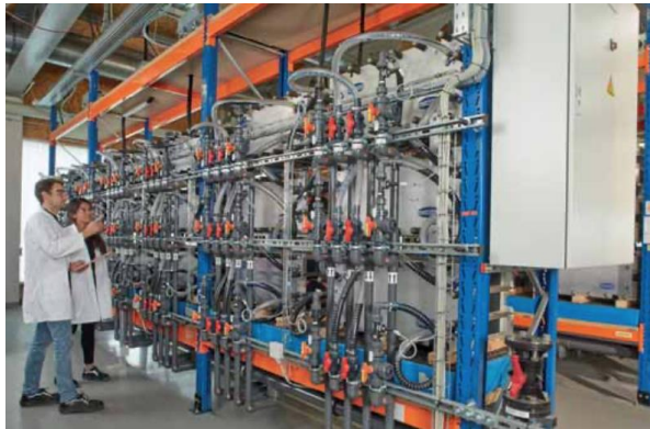
Stacks of a 2MW/20MWh vanadium redox flow battery at Fraunhofer ICT. Image:
