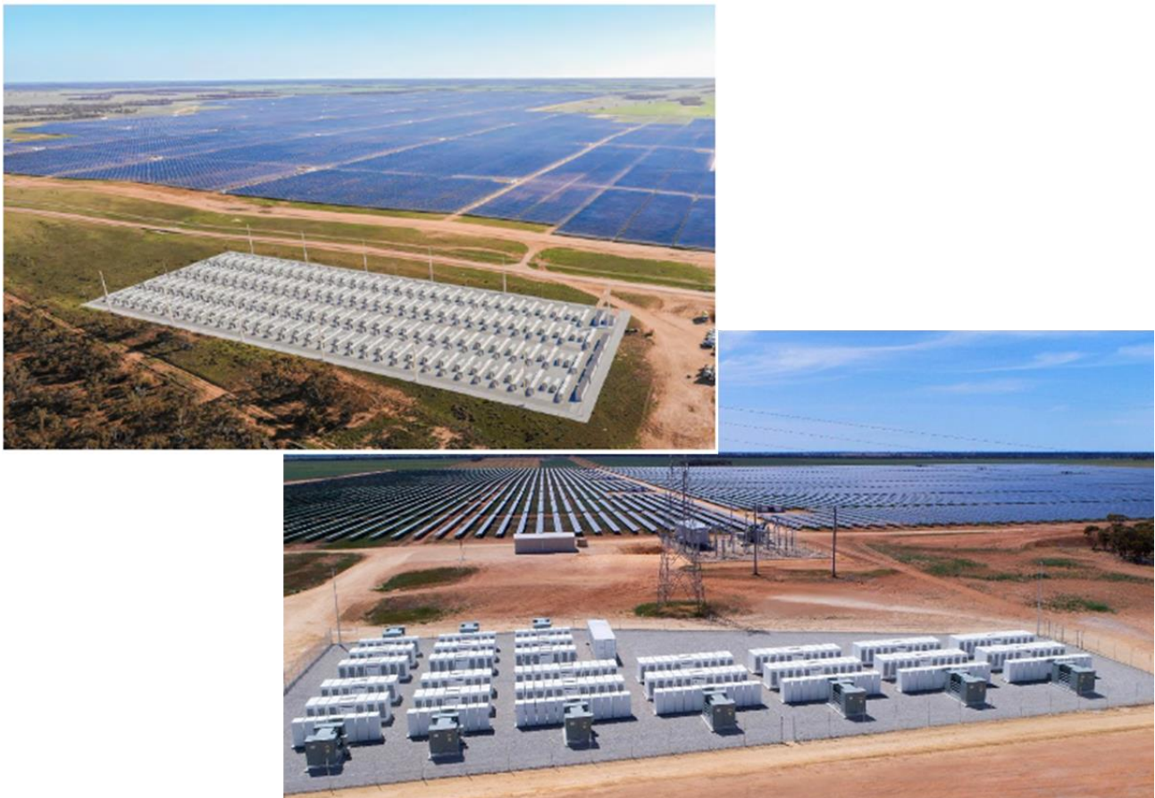
FIGURE 15.2.3.1.1 – Images of Typical BESS Systems Servicing Solar Power Farms
