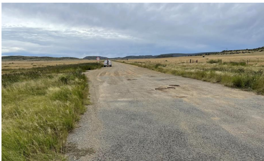
Figure 2.9: Potential Access Route Option 1: Divisional Road 3093 (Photograph taken from the R48) (Sturgeon, 2023).
