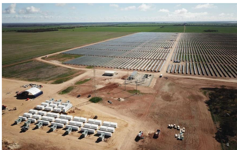
Figure 2.6. Example of PV Technology with Lithium Ion BESS (ARENAWIRE, 2018 5 ).
