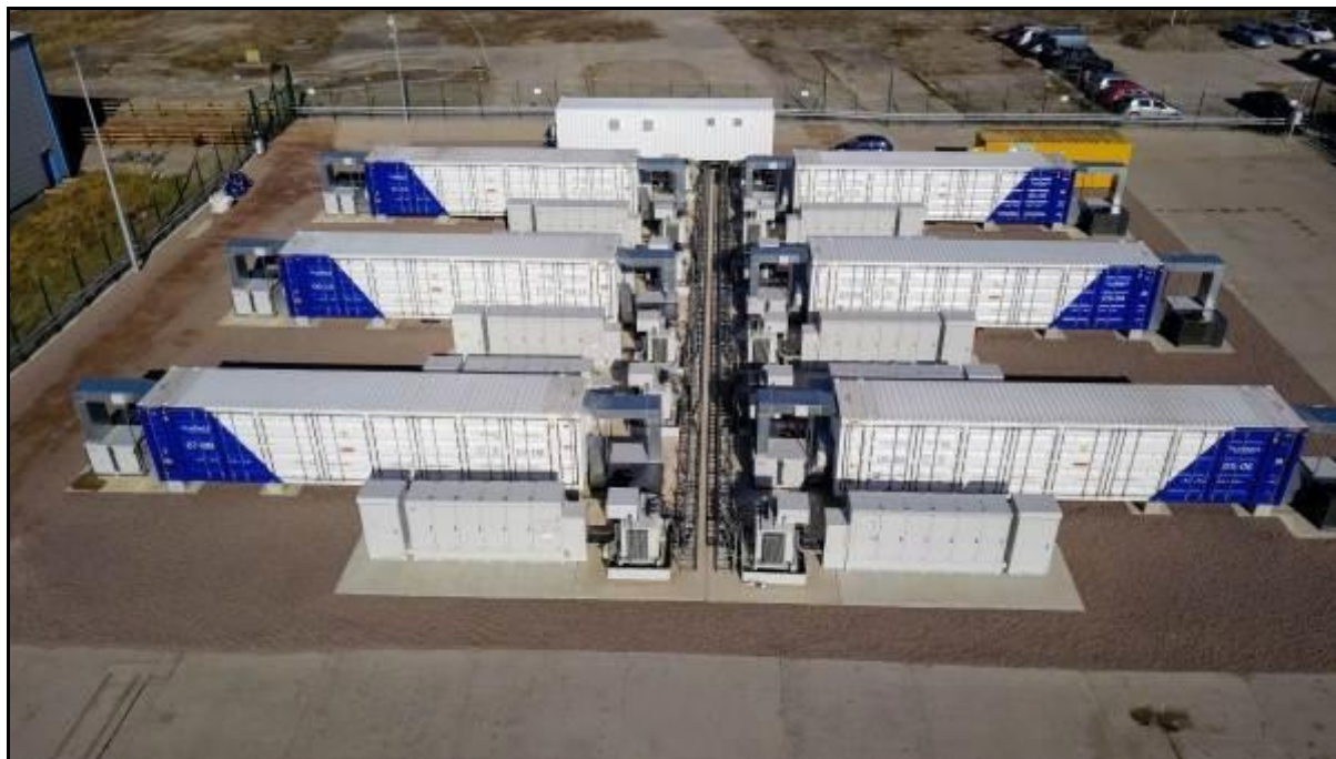
Photograph 1.2: Example of BESS located in storage containers
