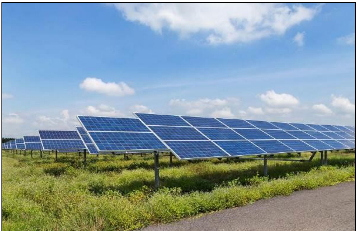
Photograph 1.1: Typical PV SEF facility
