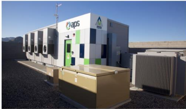
Arizona utility APS has grounded its energy storage operations while the investigation continues.
