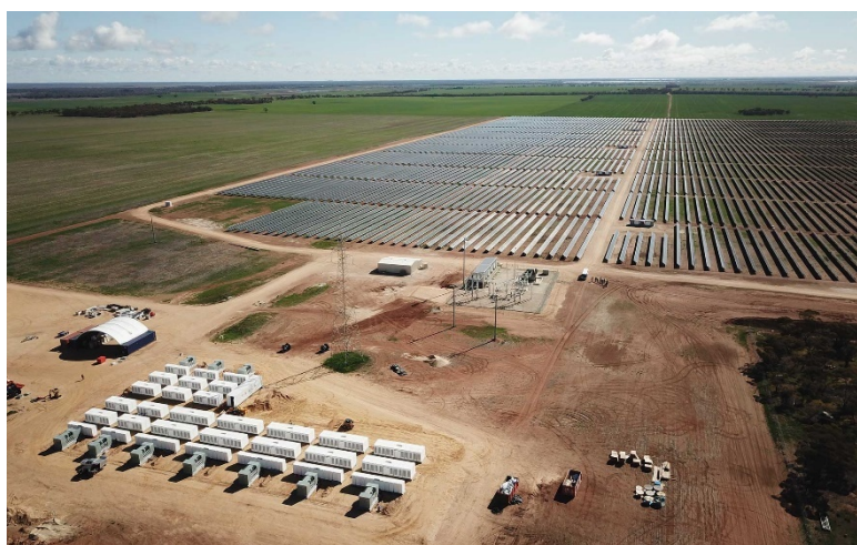
Figure 2.6. Example of PV Technology with Lithium Ion BESS (ARENAWIRE, 2018 4 )
