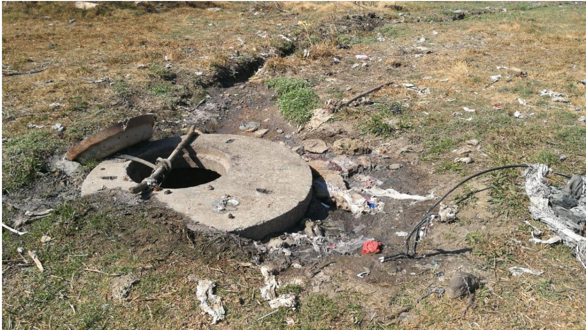
Figure 2: Vandalism of the sewerage
