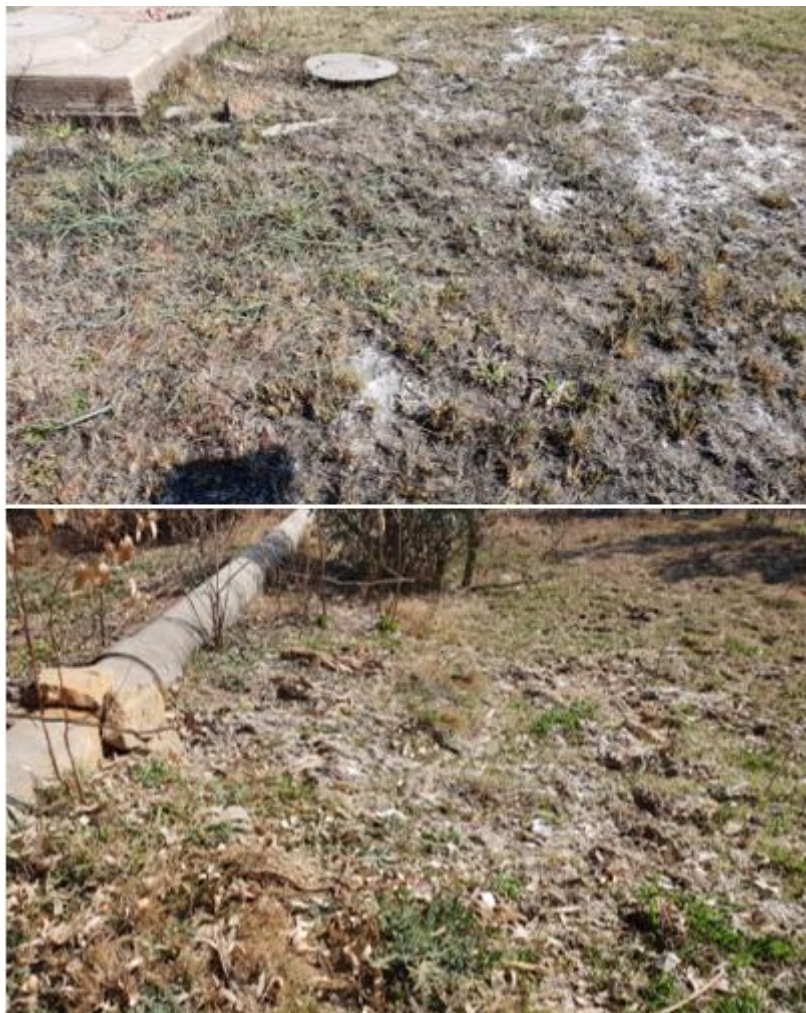
Figure 5: Sewage spillage from the pipeline
