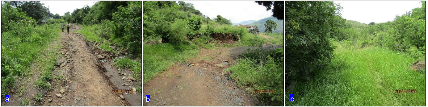
Figure 6: (a) The current access road is narrow and badly eroded. (b) An overview of where the current drainage line flows over the road and where the new culvert will be located in the watercourse. (c) A view of the upstream conditions in the riparian area above the proposed culvert location.
