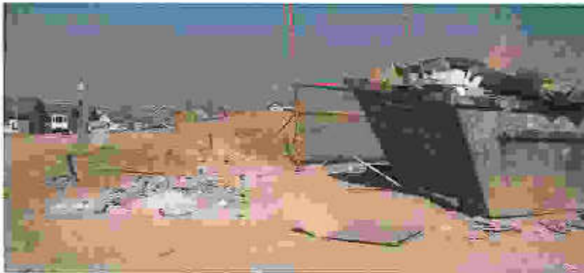
Figure 9: Waste management on site does not adhere to EMP requirements
