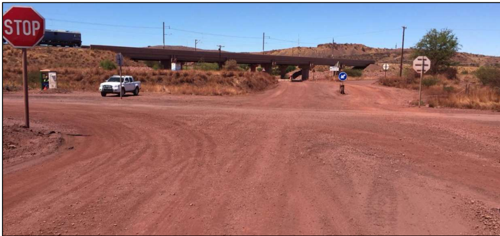
FIGURE 10-1: HAUL ROAD AND DR3333 CROSSING – LOOSE MATERIAL ON SURFACE
