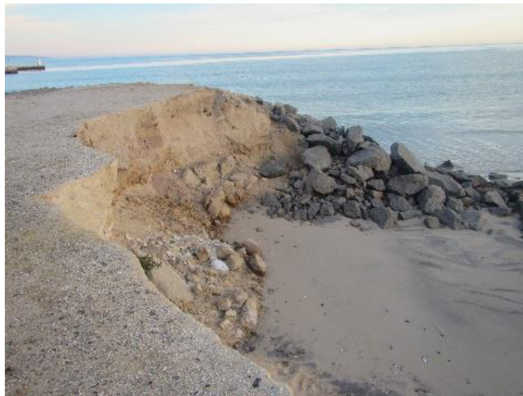
Figure 3-5 View from the top of the eroded cliffs towards the shore armouring
