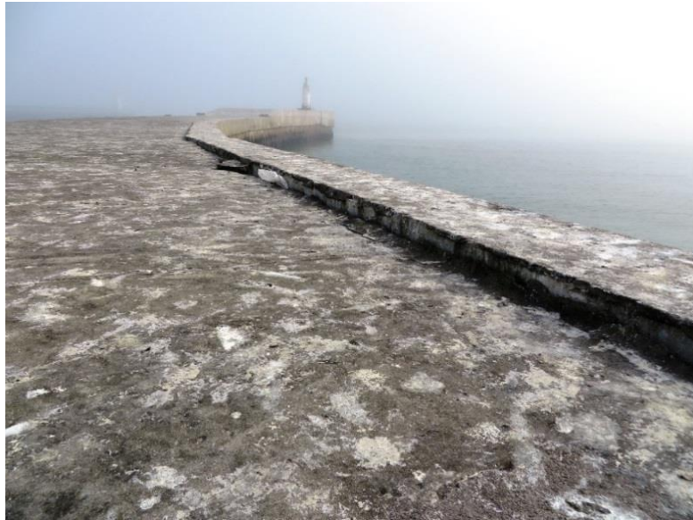
Figure 2-8 Evidence of Concrete Deck Settlement on the Eastern Breakwater
