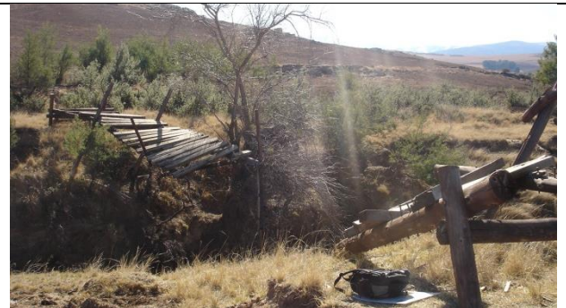
Figure 2. Image looking north towards the village of Matewu showing the collapsed pedestrian bridge that is proposed for replacement.
