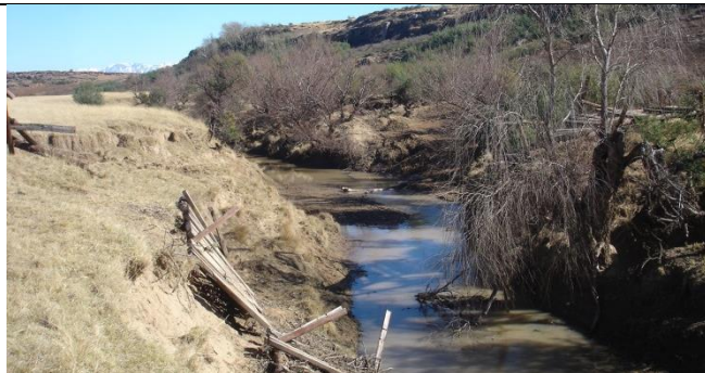
Figure 1. Image looking west showing the collapsed pedestrian bridge that is proposed for replacement.
