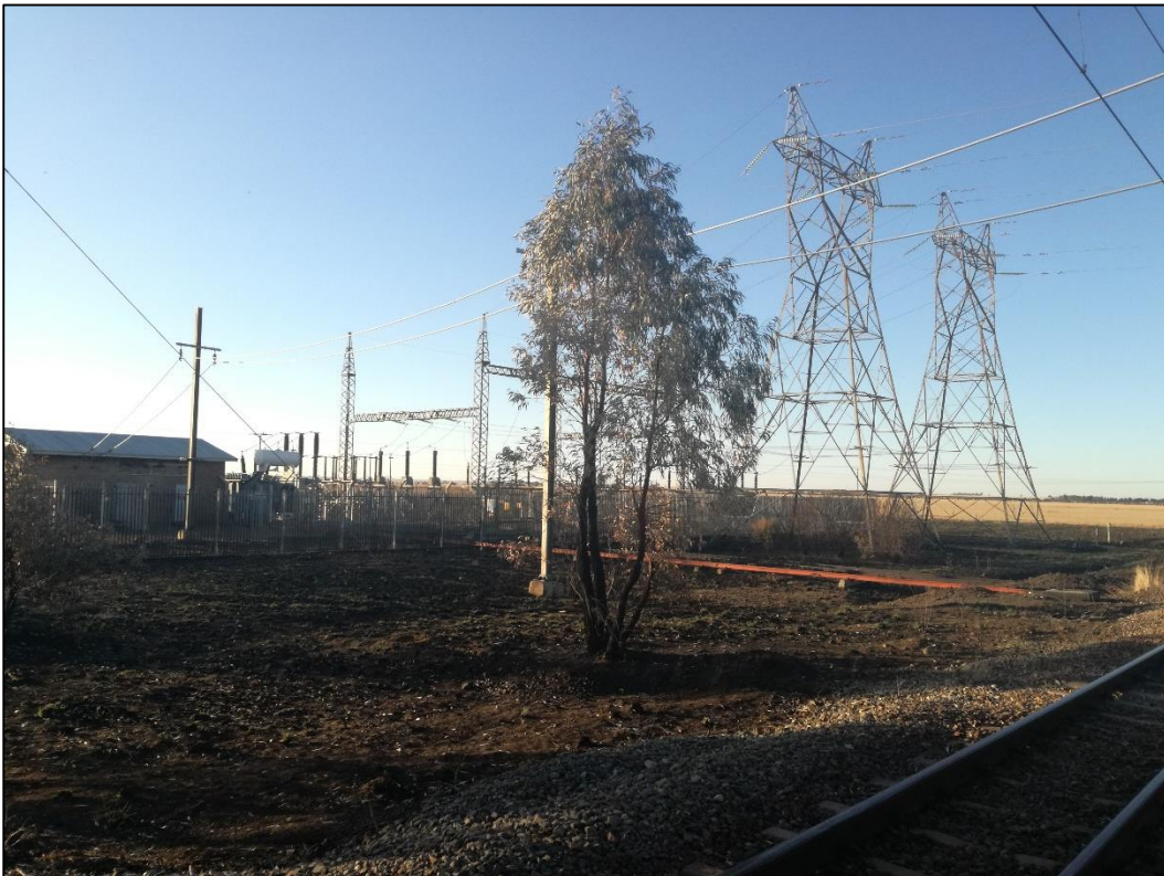
Figure 17: Power lines feeding into the Leeubos TR 132kV Traction Substation
