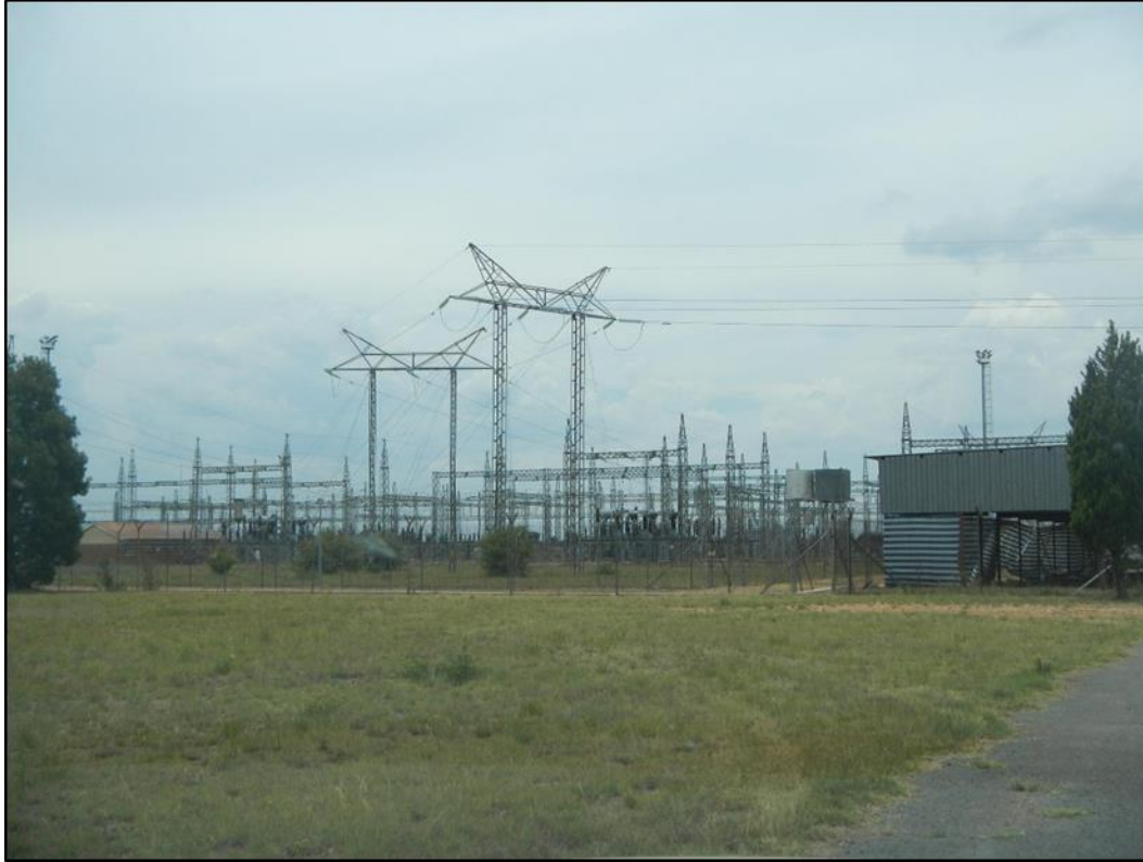
Figure 48: Watershed Substation near Lichtenburg in the North West Province is a good example of a typical Eskom Substation
