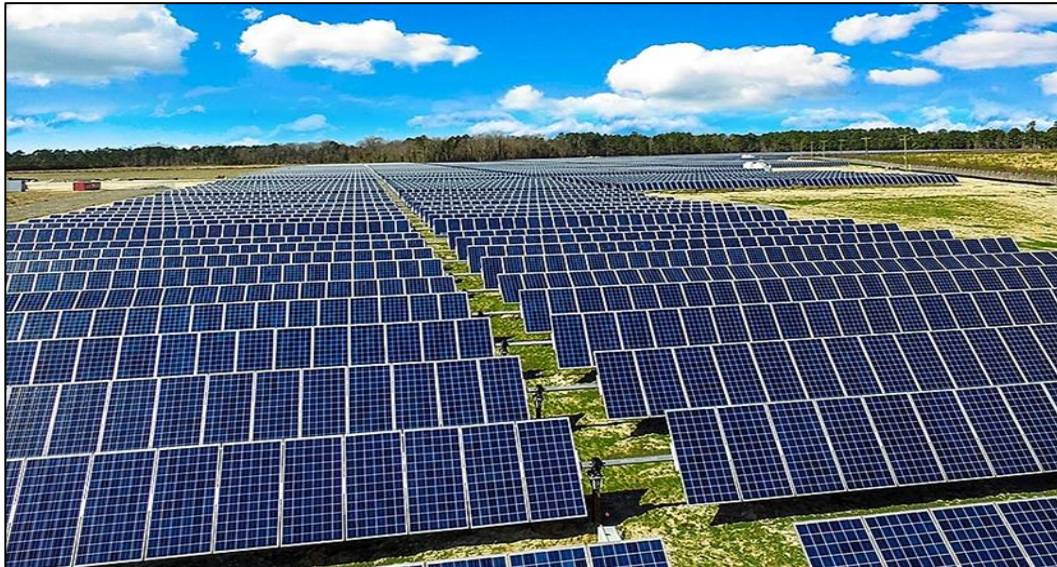
Figure 2.1: Typical example of solar PV array
