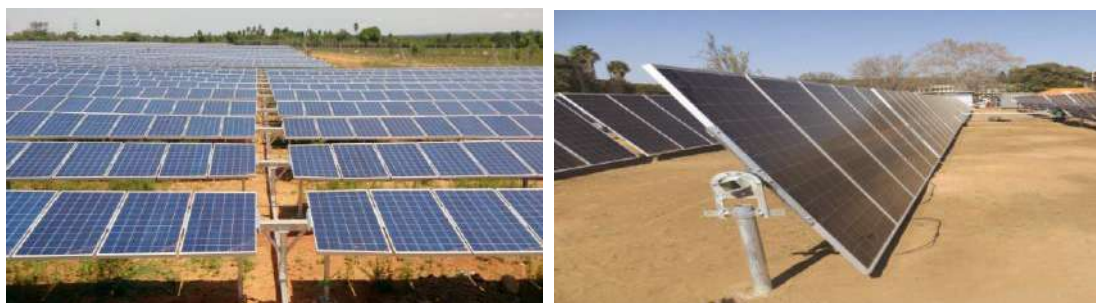
Figure 2-1: Single axis solar PV module tables raised 1.5m above ground level (to a maximum tilt height of 3m)
