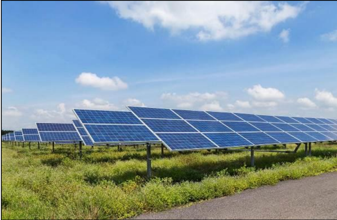
Photograph 1.1: Typical PV SEF facility
