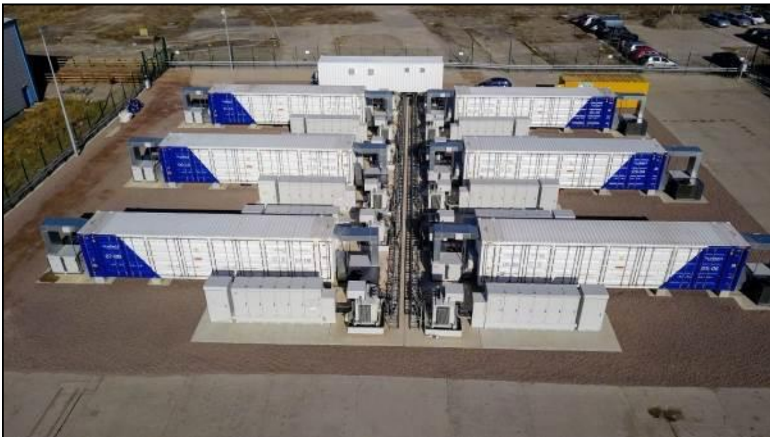
Photograph 1.2: Example of BESS located in storage containers
