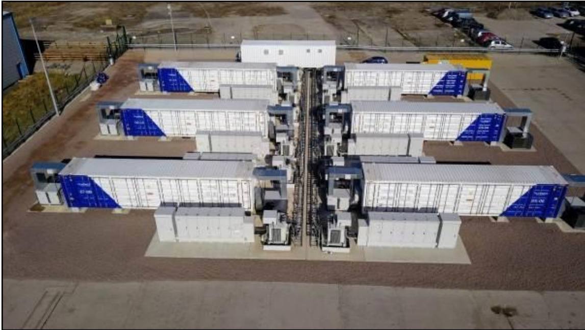
Photograph 1.2: Example of BESS located in storage containers
