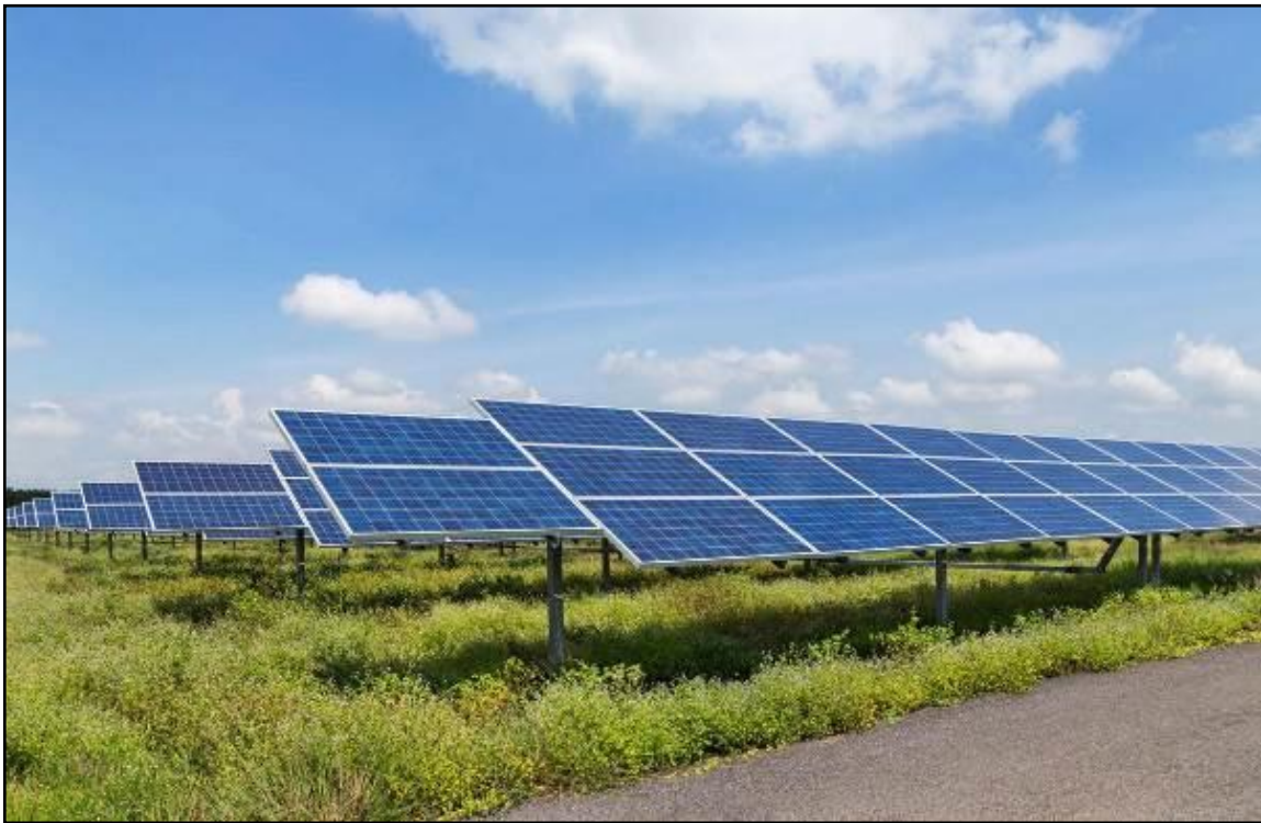
Photograph 1.1: Typical PV SEF facility
