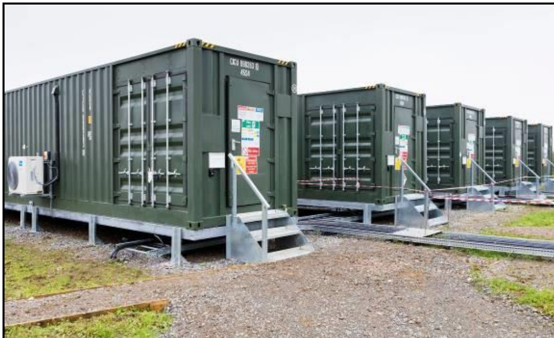
Photograph 1.2: Example of BESS located in storage containers
