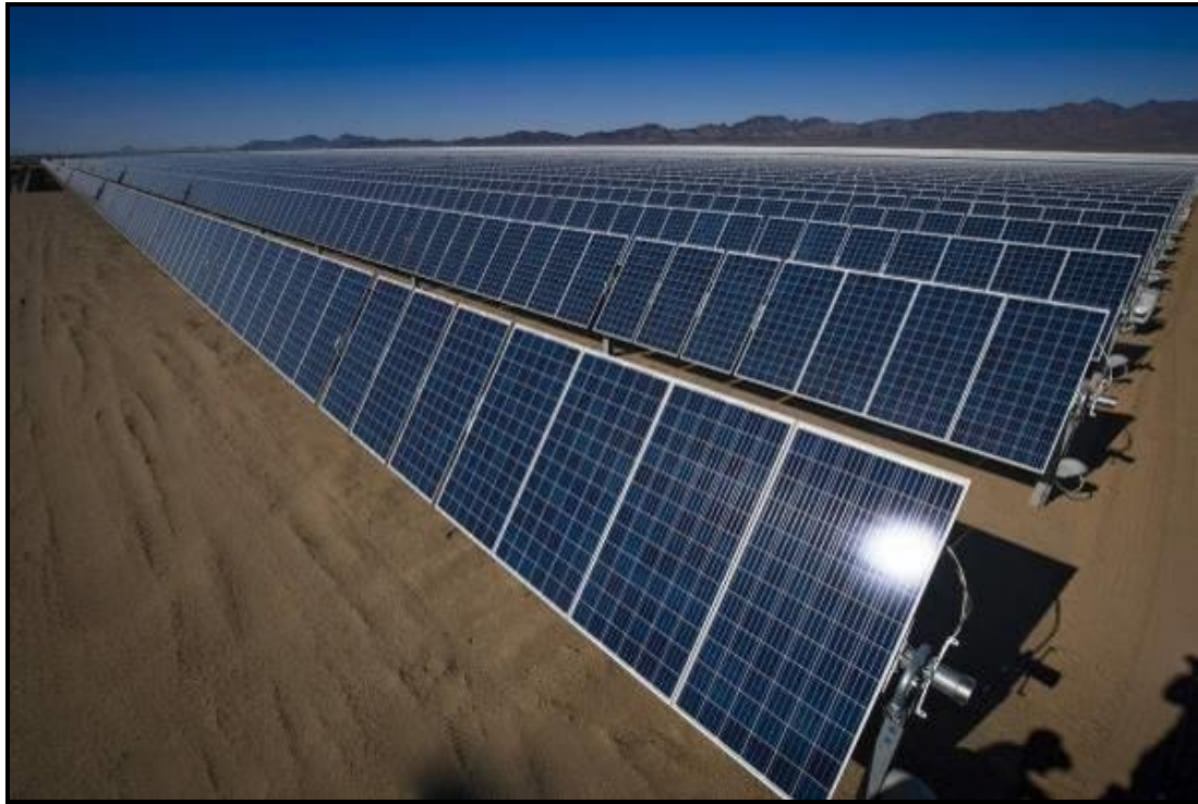
Photograph 1.1: Typical PV SEF facility
