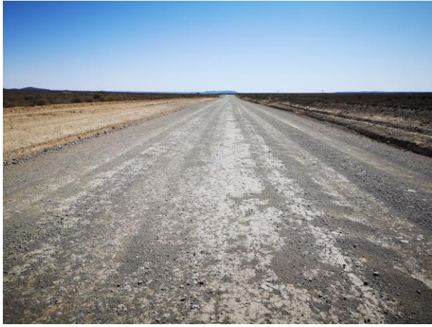
Image 5-5 Typical condition of AP2972
