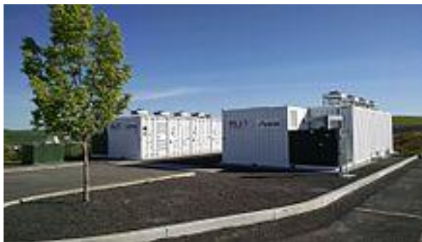
FIGURE 2.3.2.1 – Images of Some Redox Flow BESS Systems – containerized systems or buildings with tanks of electrolyte and battery systems
