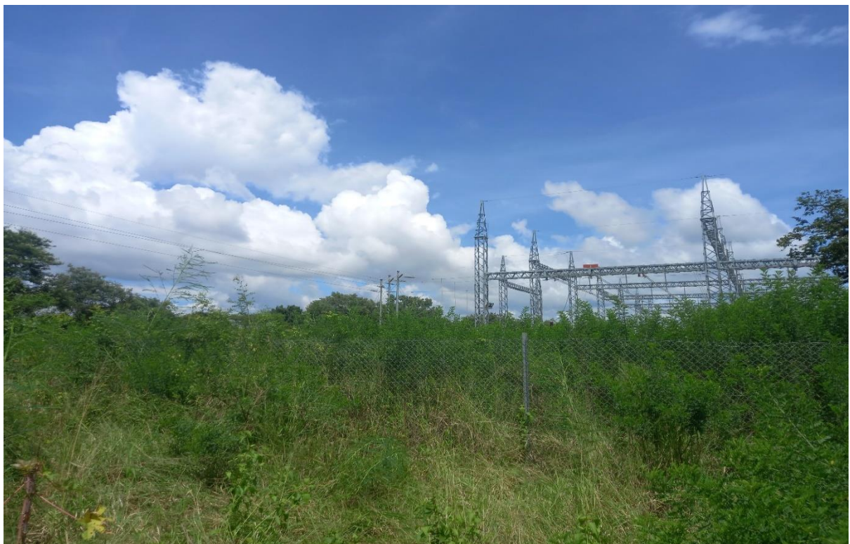
Figure 3: Another view of the proposed development showing the existing powerline at Letaba.
