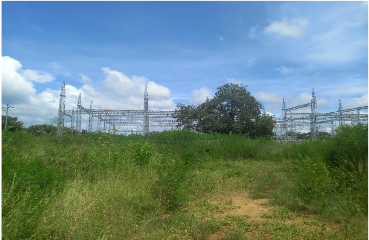
Figure 2: General site overview of the substation at Letaba.
