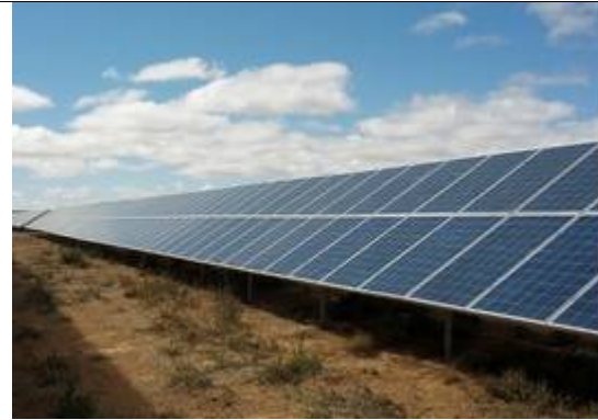
Figure 2.2: Picture of a PV Modules (75 MW plant in Kalkbutt South-Africa Source: SMA)
