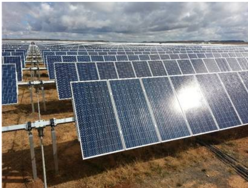
Figure 2.6: The support structures elevate the PV panels and allow for single axis tracking of the sun for increased efficiency (Source: SAPVIA)
