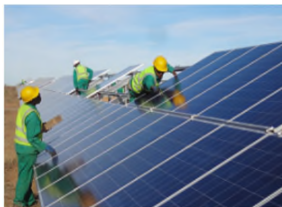
Figure 2.4: Picture of the installation of a typical PV array (75 MW plant in Kalkbutt South-Africa Source: PennEnergy)
