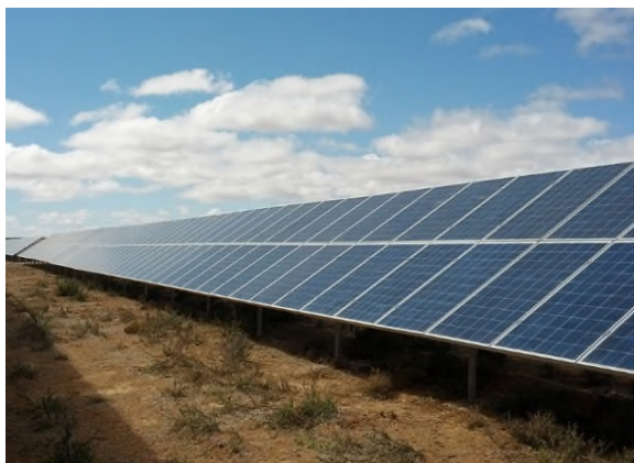
Figure 2.3: Picture of a PV Modules (75 MW plant in Kalkbutt South-Africa Source: SMA)
