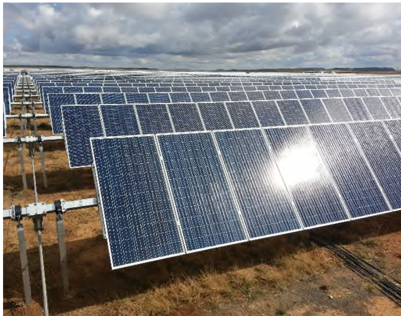
Figure 2.7: The support structures elevate the PV panels and allow for single axis tracking of the sun for increased efficiency (Source: SAPVIA)
