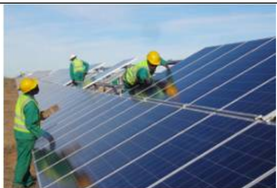
Figure 2.3: Picture of the installation of a typical PV array (75 MW plant in Kalkbutt South-Africa Source: PennEnergy)
