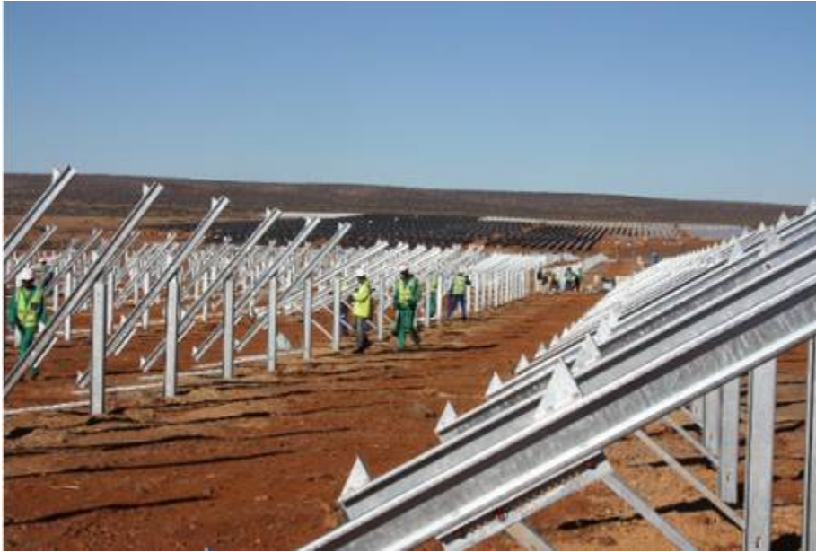
Figure 2.7: Frame, structural details (Lesedi Solar PV Project, Kimberly, South Africa. Source: Power Technology.com)
