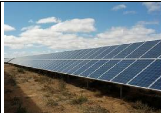
Figure 2.2: Picture of a PV Modules (75 MW plant in Kalkbutt South-Africa Source: SMA)
