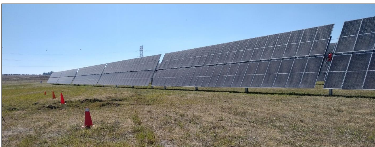
Figure 5. Front views of the PV arrays mounted on horizontal 1-axis tracker
