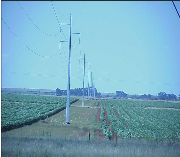
Figure 1: Example of the Monopole Tower Type
