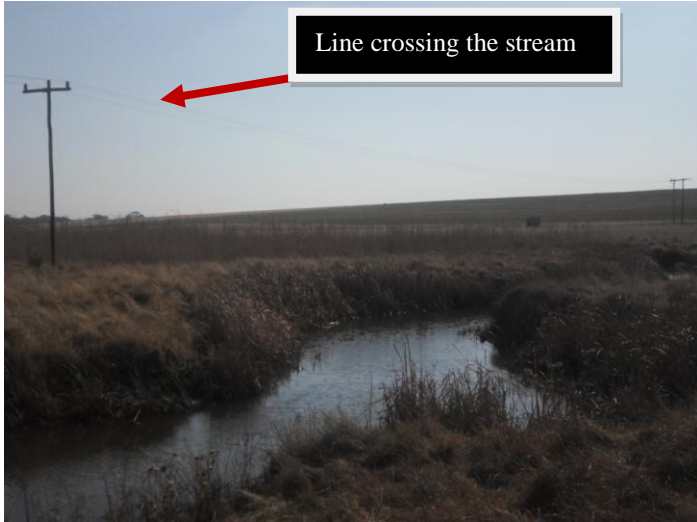
Image 2: Line crossing at farm Maresrust 515
