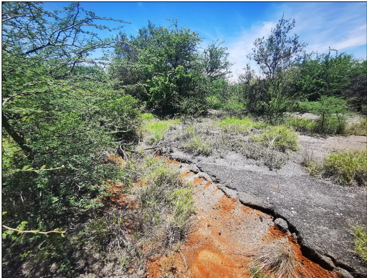
Figure 32: Illustration of concrete within the bed of the tributary
