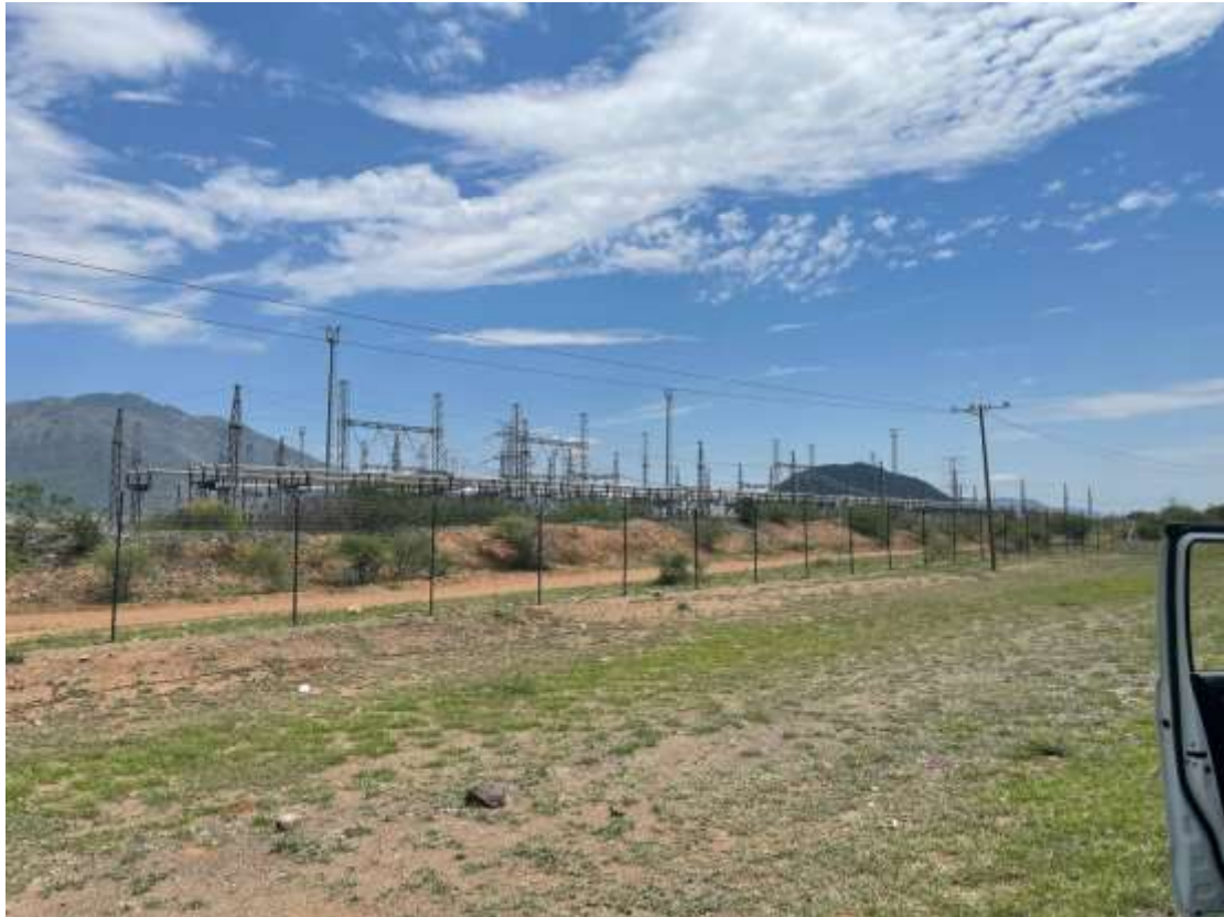
Figure 14: Low VAC at the Senakangwedi Substation.
