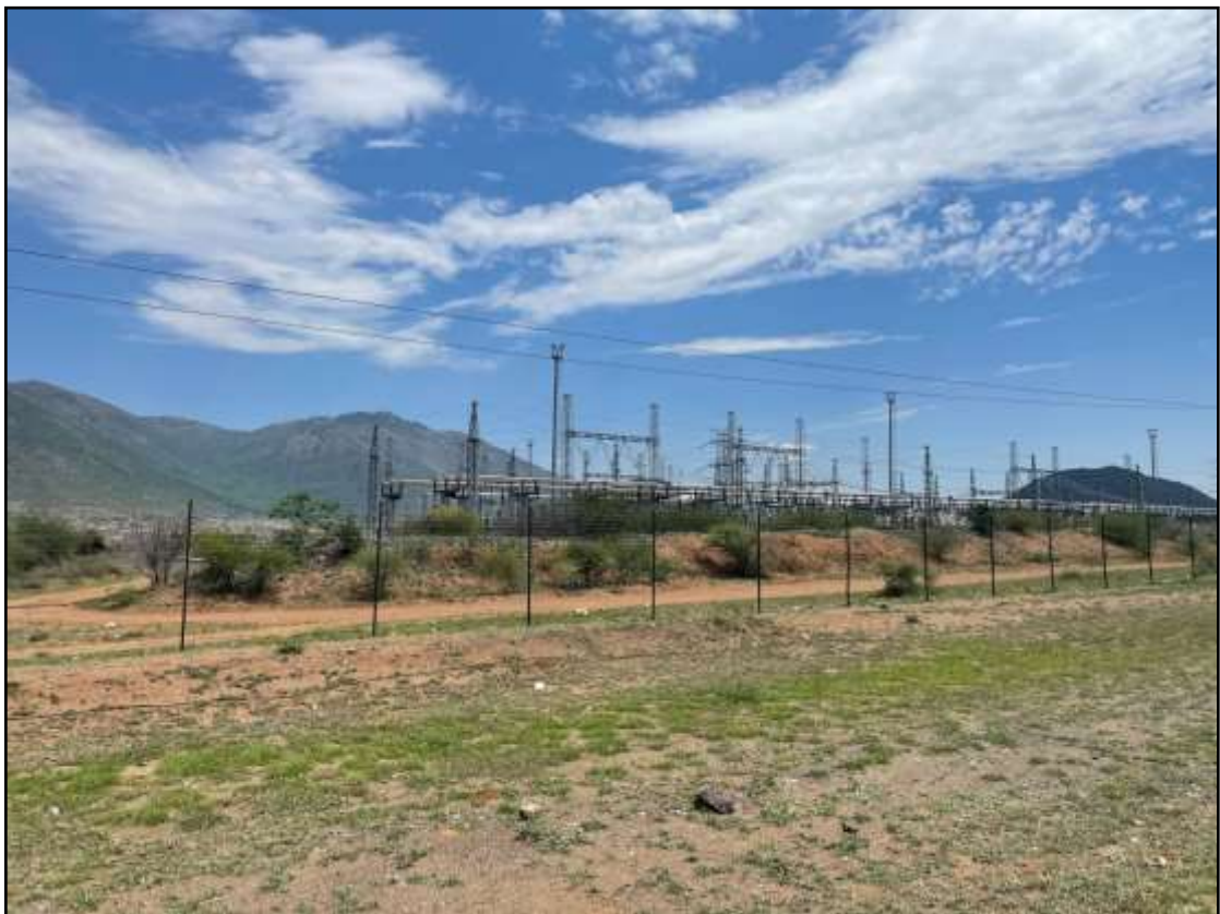
Figure 11: The Eskom Senakangwedi 275/33kV Substation.
