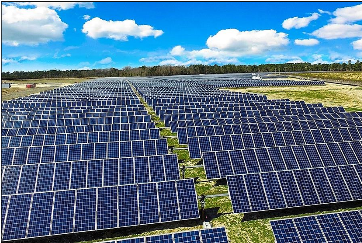
Figure 2.1: Typical example of solar PV array
