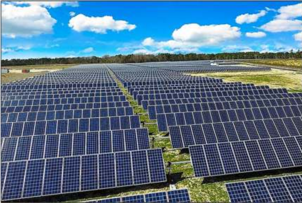
Figure 2.1: Typical example of solar PV arrays
