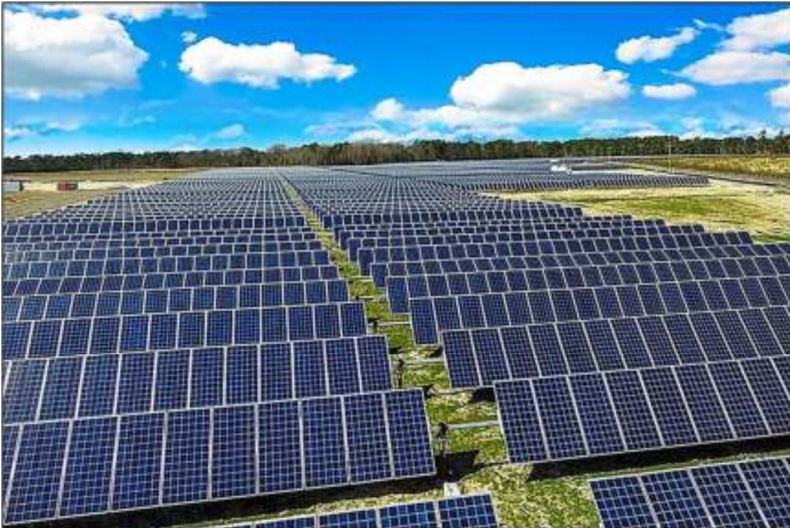
Figure 2.1: Typical example of solar PV arrays
