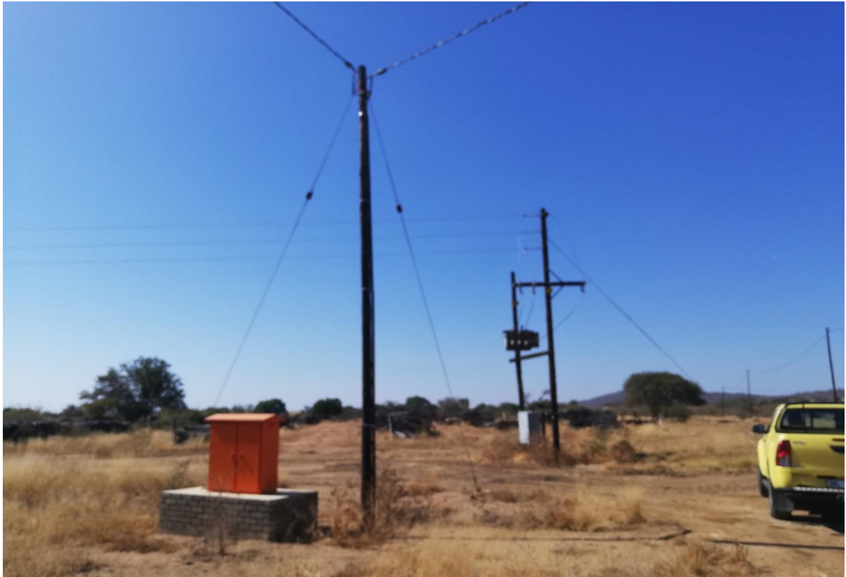
Pictures showing the existing powerlines in the ZZ2 Farm
