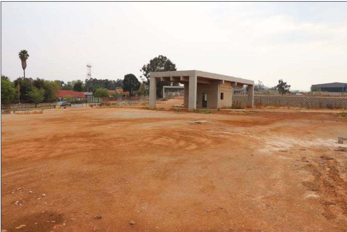
Figure 12 – The partially completed main entrance gate located at the southern end of the study area can be seen in this image. Notice the terracing on the right.
