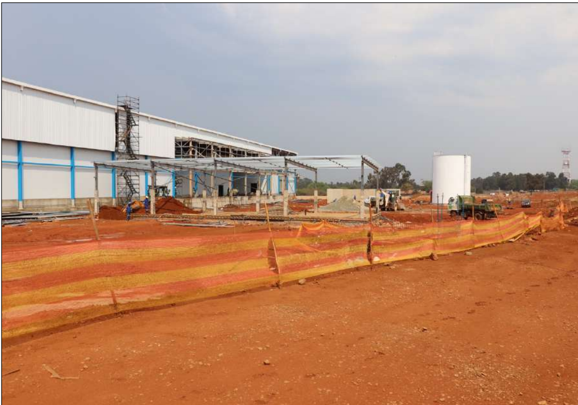
Figure 10 – General view of a section of the study area. The site is currently undergoing construction work
