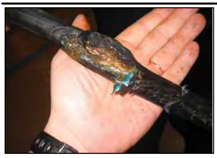
Figure 9.8 Photograph of cable damaged by a grapnel intended to retrieve fish traps from 1800 m depth.
