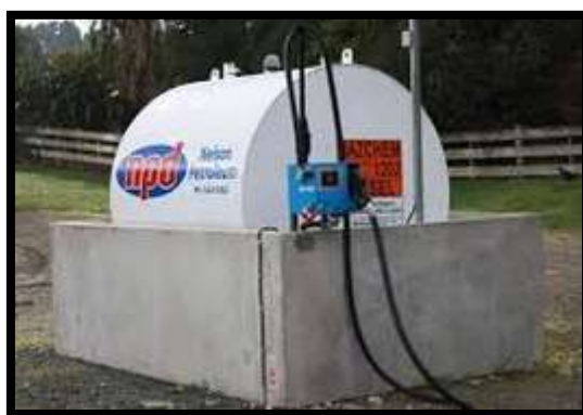
Figure 27: Typical surface fuel storage tank with bunding
