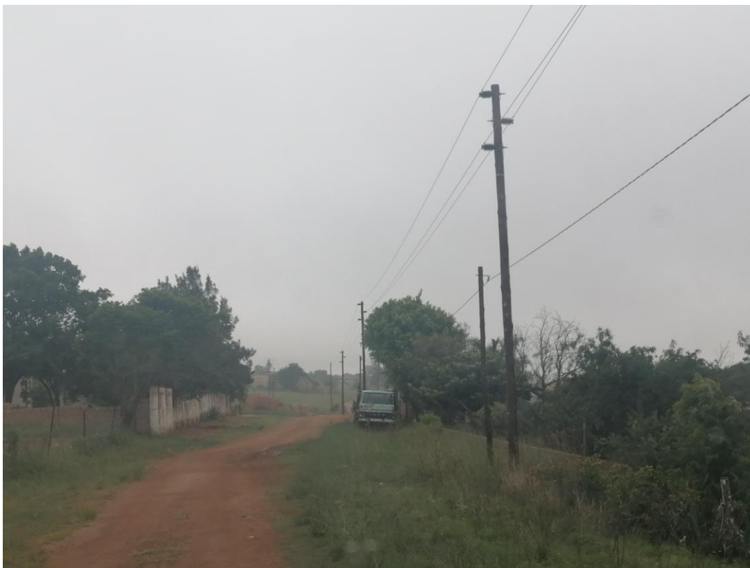
Photo 2: Shows the existing powerlines on site
