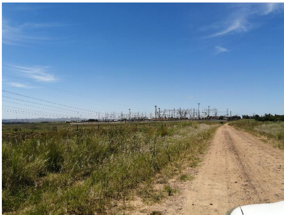
Figure 11: Incandu switching station
