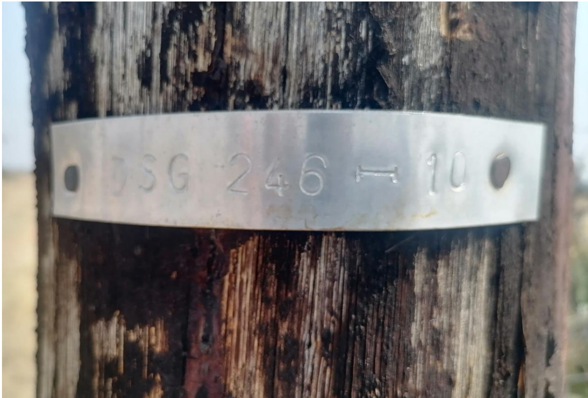
Photo 1: Shows the existing pole number on site
