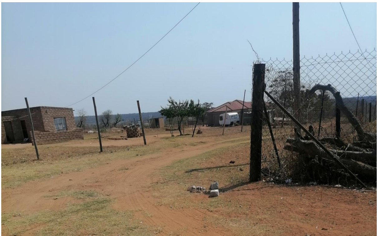
Photo 6: Shows the peg on site where the new pole will be planted 3
