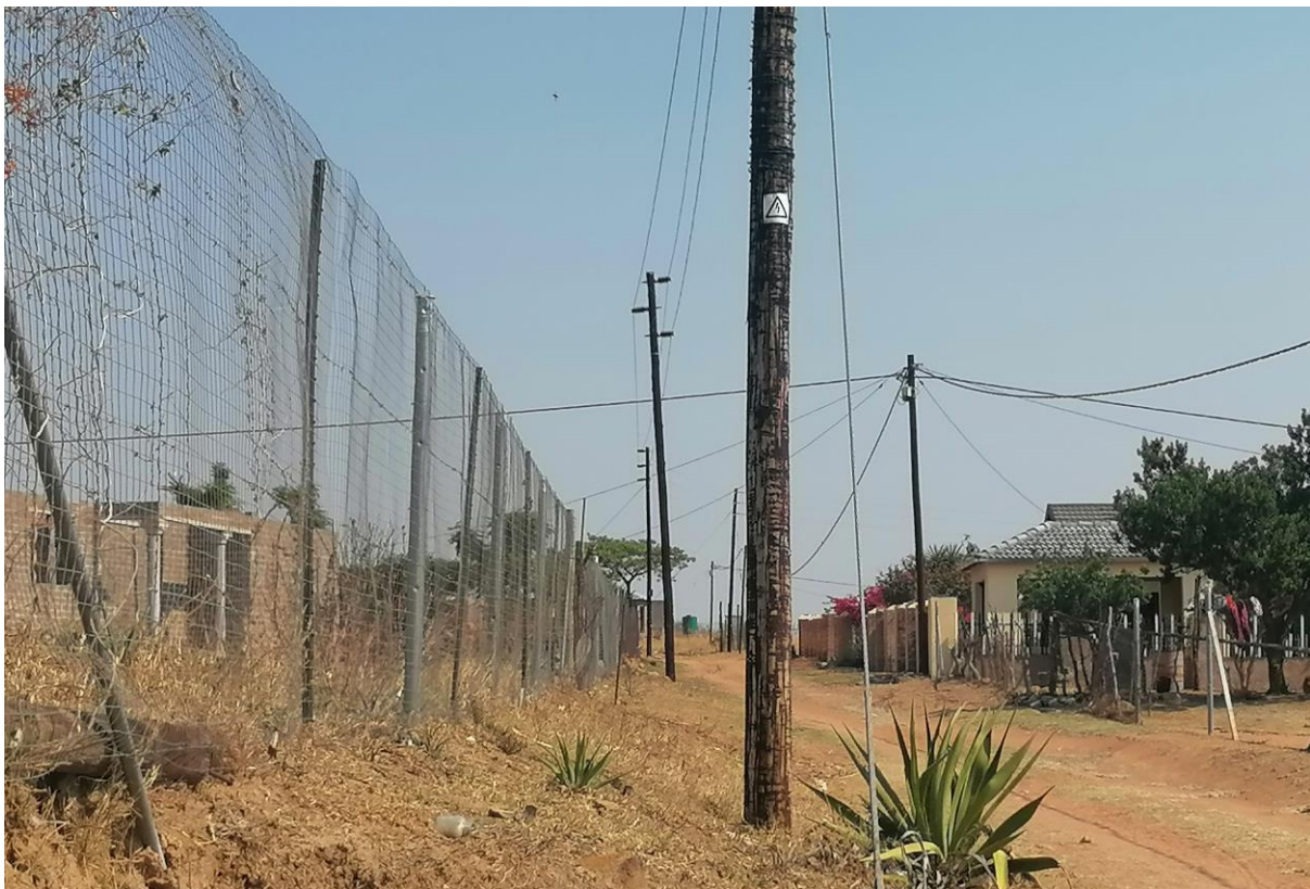
Photo 2: Shows the existing powerline on site
