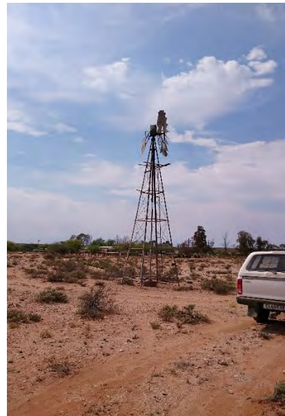
BH6 - wind pump
