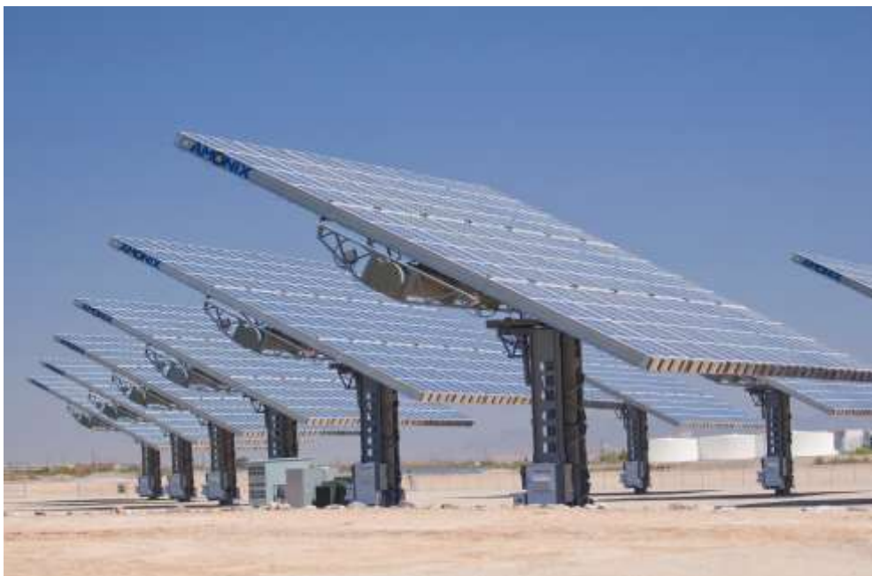
Figure 3.3: The support structures elevate the panels by 16 m and allow for dual axis tracking of the sun for increased efficiency (Source of Amonix™).
