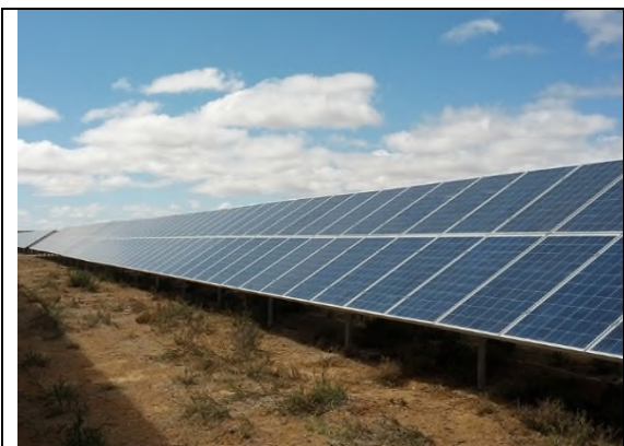
Figure 2.3: Picture of a PV Modules (75 MW plant in Kalkbutt South-Africa Source: SMA)
