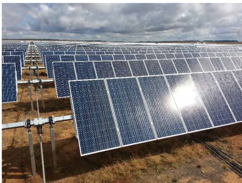
Figure 2.7: The support structures elevate the PV panels and allow for single axis tracking of the sun for increased efficiency (Source: SAPVIA)
