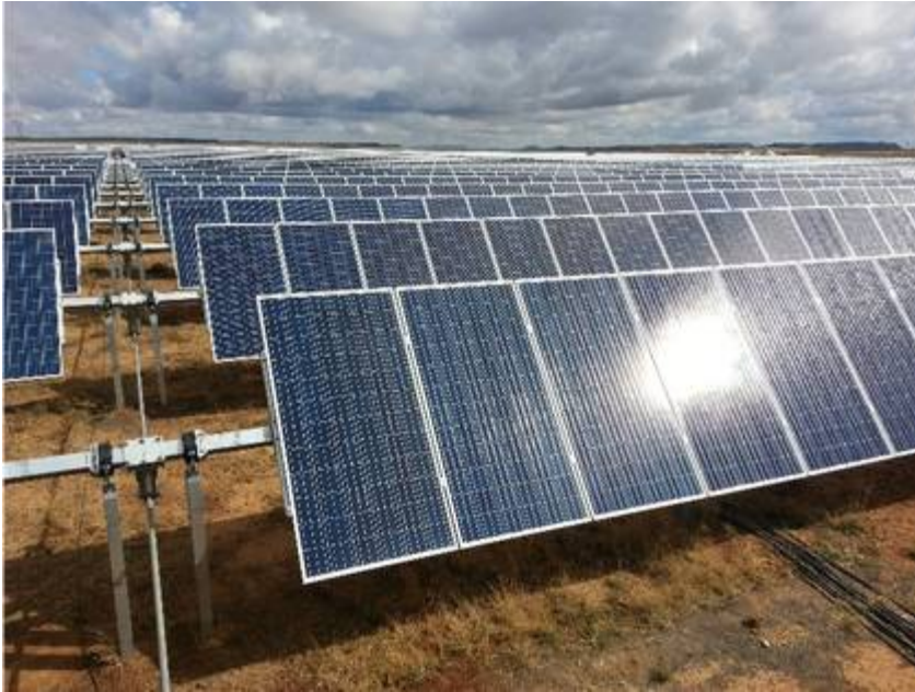
Figure 2.6: The support structures elevate the PV panels and allow for single axis tracking of the sun for increased efficiency (Source:SAPVIA)
