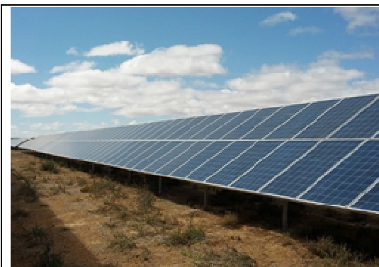
Figure 2.2: Picture of a PV Panel Modules (75 MW plant in Kalkbutt South-Africa Source: SMA)
